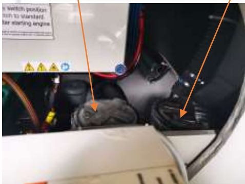
Generator raw water strainer
