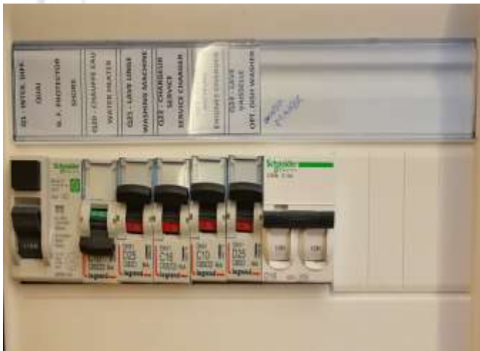
Top row of breakers (Chargers and Water Heater)
