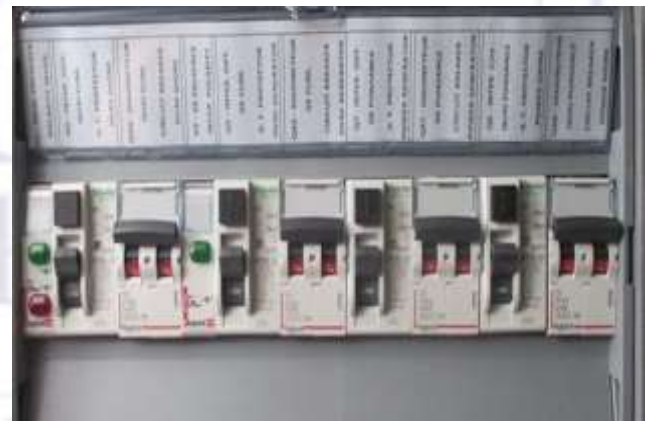
Main 110V breakers in port eng room
