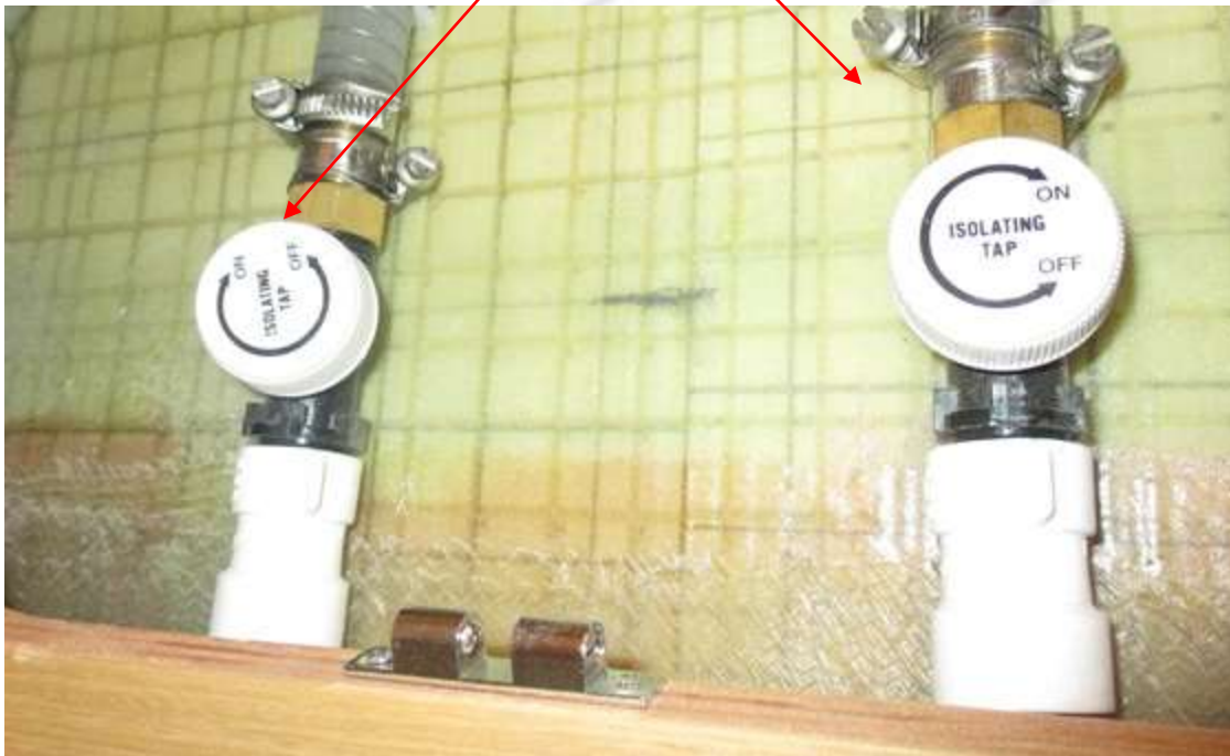
Water tank valves
