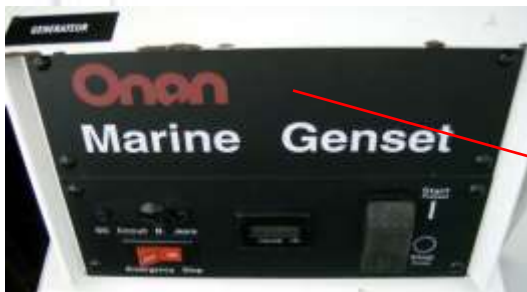
Main breakers for the generator
