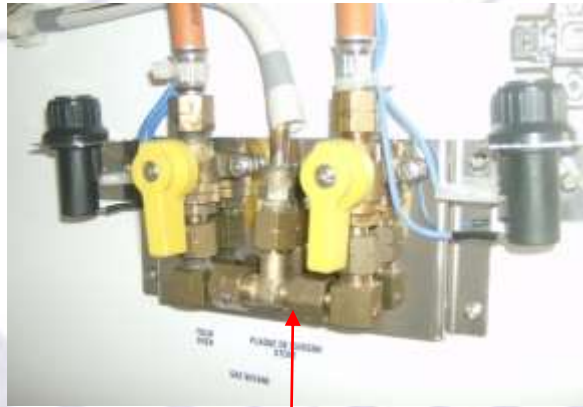
Gas shut off valves under sink
