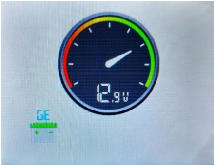
Generator battery voltage
