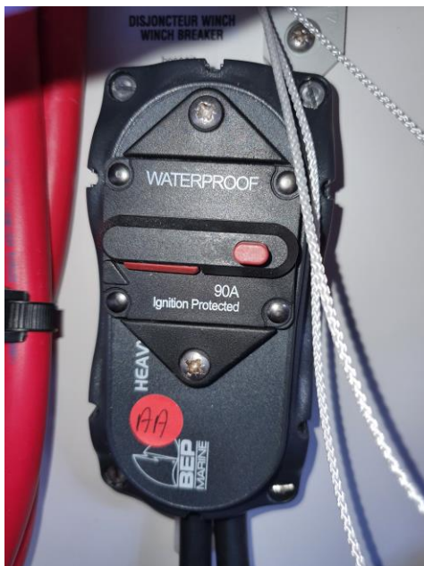
Davit Winch Breaker
