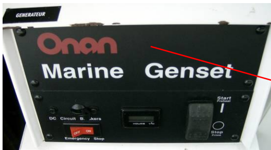
Main breakers for the generator
