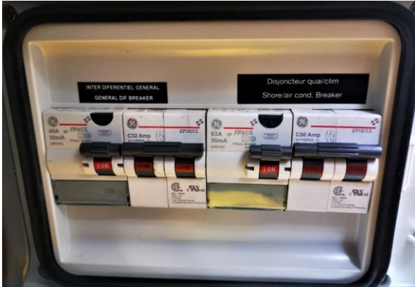
Main shore power breakers
