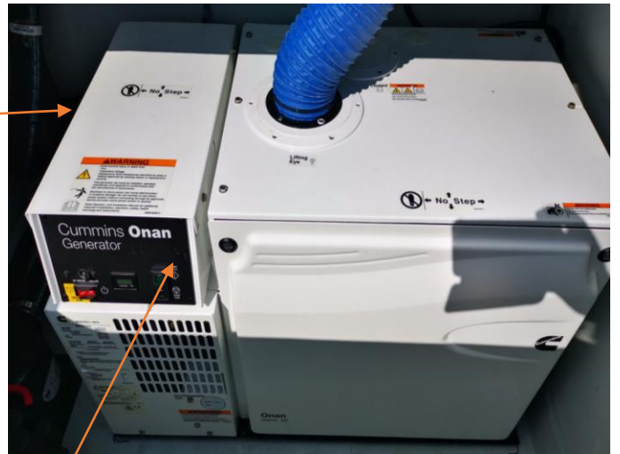
Cummins Onan Generator
