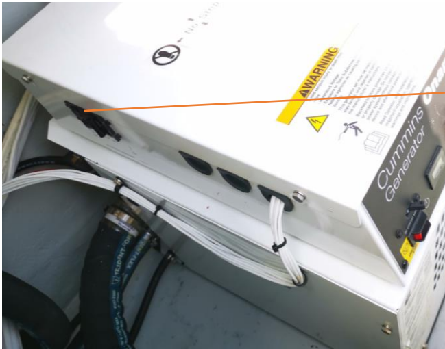
Generator Reset Breaker
