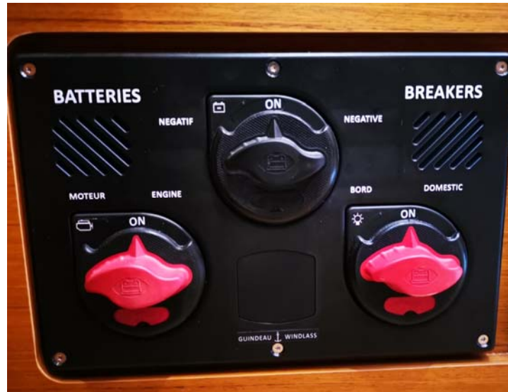
Domestic (Main) Battery Switch
