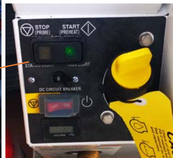
Generator Start panel
