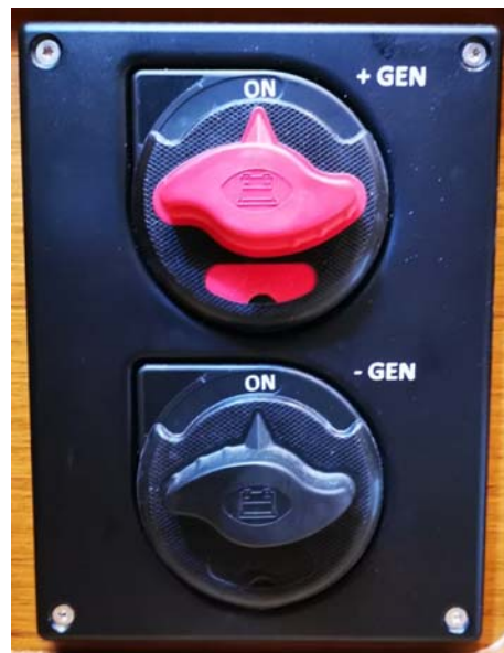
Generator Battery Switch
