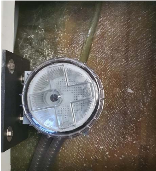
Generator raw water strainer, STBD midship floorboard
