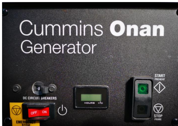
DC Circuit Breakers, Emergency Stop, Hour meter and Start/Stop (Prime)
