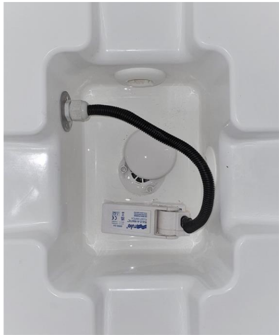
Shower Drain with Automatic Float Switch
