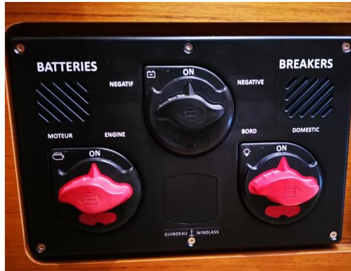
Domestic (Main) Battery Switch
