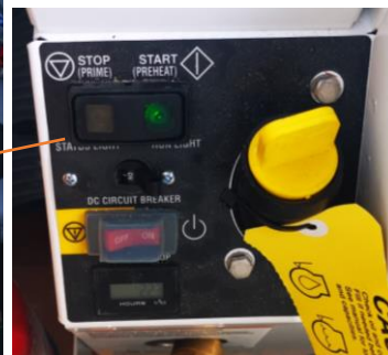
Generator Start panel
