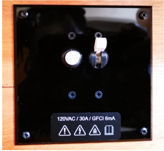
If electrical outlets are inoperable, please reset the GFCI Breaker.
