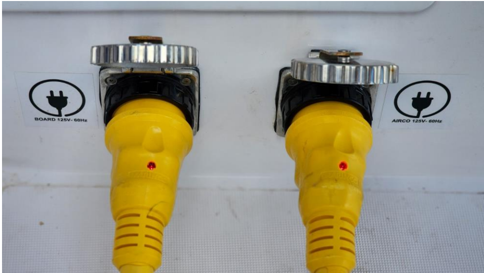
Shore power air conditioning
