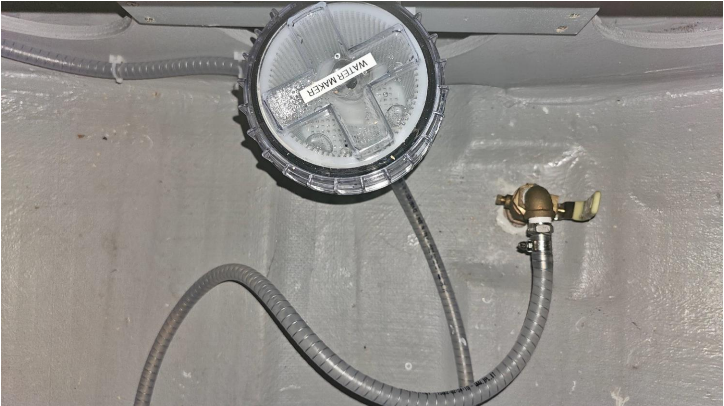
Watermaker intake valve and strainer below starboard fwd cabin floorboard
