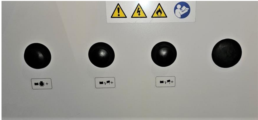
Shore power charger and outlets
