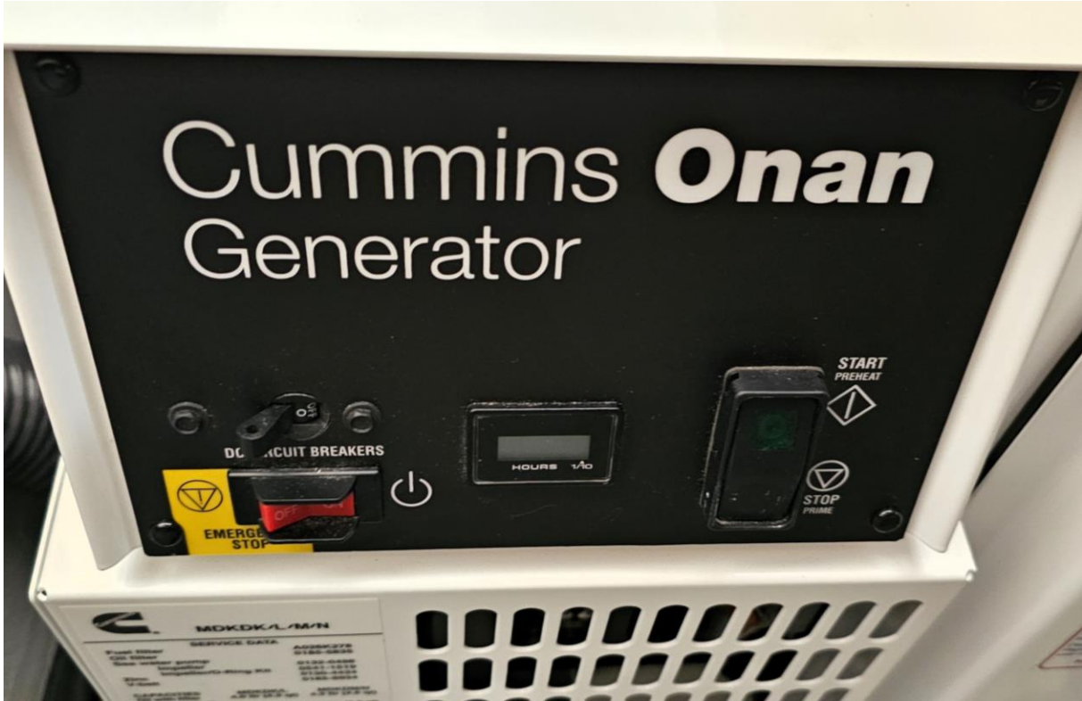
Generator Control Panel
