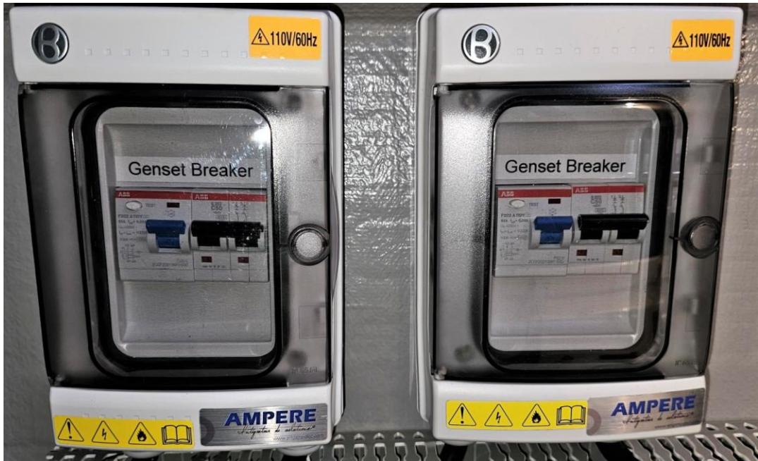
Generator Breakers Below Starboard Aft Bunk
